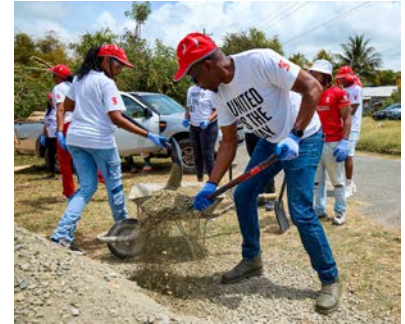
Scotiabank Tobago employees supported with the installation of a rainwater harvester in the community of Delaford for National Day of Caring 2026.
